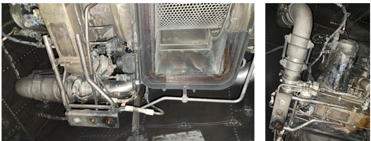
3. APU Rear Drain Oil Traces
