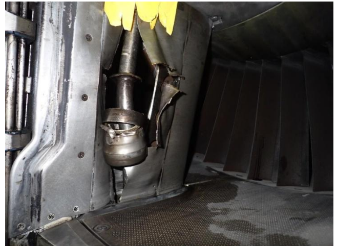
Figure 10: Fan frame strut 7 significant damage
