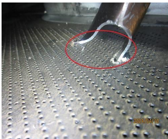
Figure 17: After acoustical panel DOD damage
