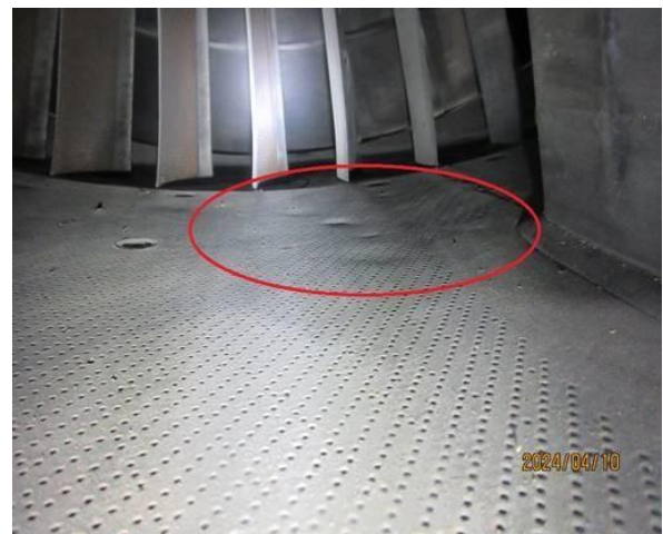
Figure 16: Middle acoustical panel impact damage
